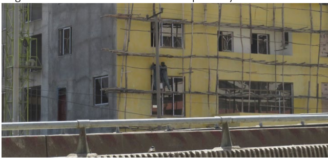
2. Construction of modern buildings also has a very distinct ancient style to it!
